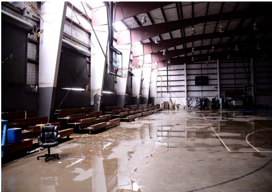
Figure 10: Structural and flood damage to the Yigo gymnasium (Credit: John O'Connor / Guam Daily Post)
